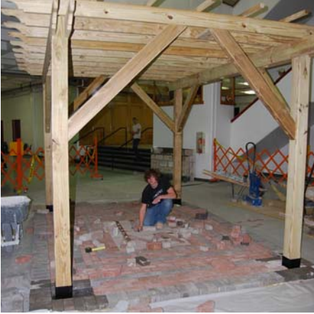
Masonry junior Matt Palmer works on the brick patio under the pergola built by carpentry students.
